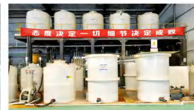
Acid process of water 制酸制水工序
