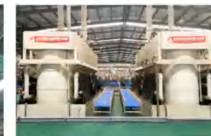
酸循环设备 Acid recycling equipment
