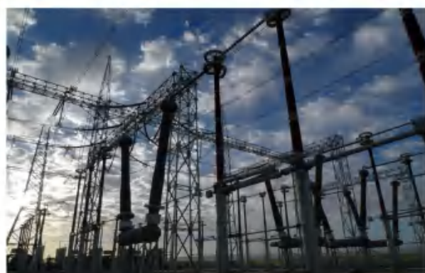
丰日蓄电池组、GZG5高频开关电源在西北电网750KV变电工程使用 Fengri accumulator and GZG5 HF switch power are applied in 750kV power transformation project of Northwest Grid.
